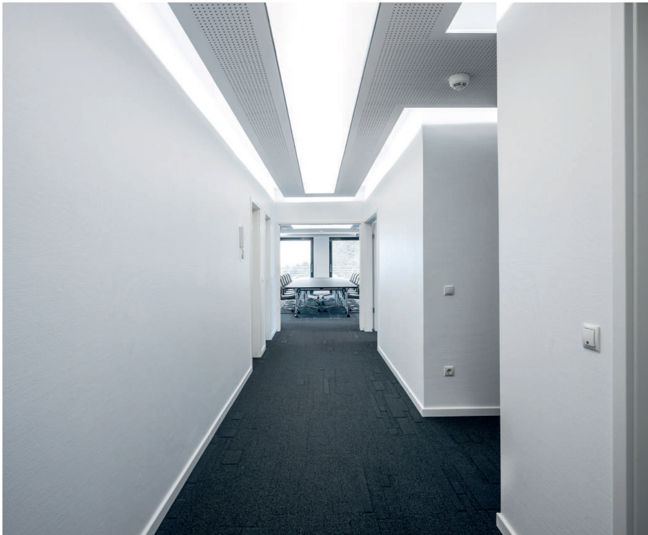
The corridors are uniformly illuminated by indirect lighting provided by QualityFlex® LED flex boards.
